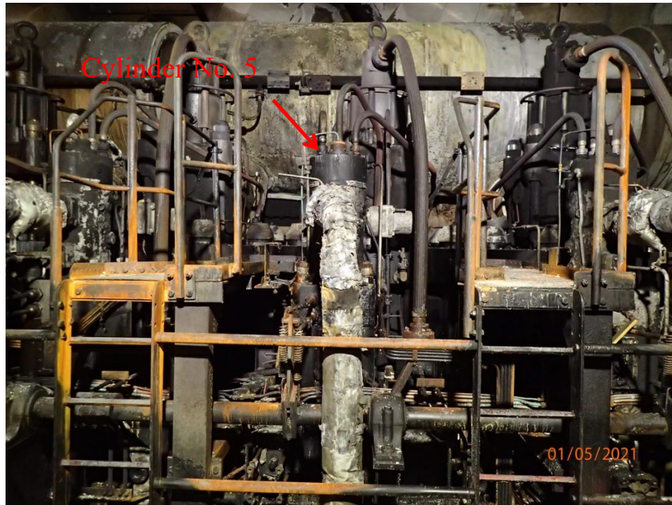
Figure 9. Side view of main engine and the initial location of the fire. (Source: U.S. Coast Guard)
