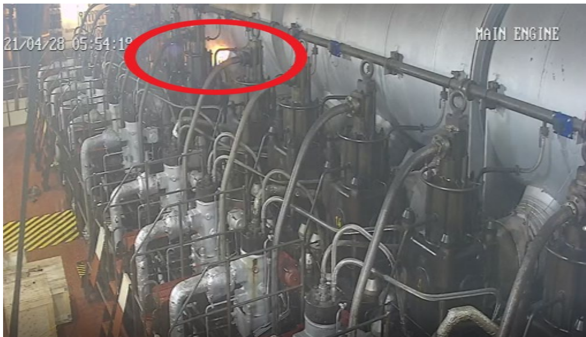
Figure 4. Screen shot of the main engine feed ships internal video recording device showing the moment the first explosion occurred at cylinder No. 5 exhaust bellows. (Source: APL)
