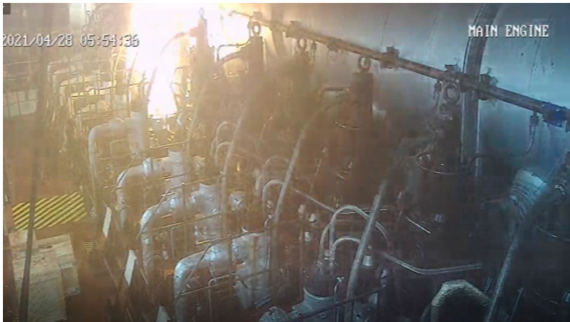
Figure 5. Screen shot of the main engine feed ships internal video recording device showing the flames spreading to cylinders 4 and 6. (Source: APL)
