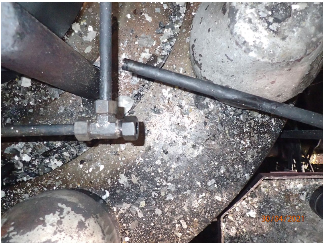
Figure 14. The fuel oil return line found separated from the T-joint. (Source: U.S. Coast Guard)
