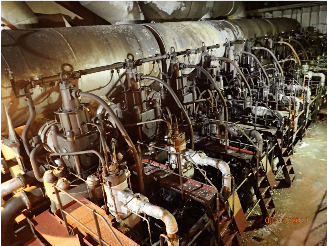
Figure 8. Photo taken on April 30, 2021 showing the fire damage to the port side of the main engine. (Source: U.S. Coast Guard)
